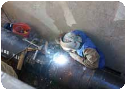
GSA HOTD Steamline Replace Project Washington, DC
